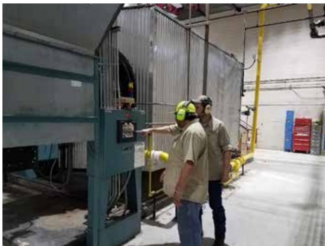
Plant Operator Hilario Villarreal with Plant Mechanic Bryan Brassell working together to ensure safe startup of Boiler 1 at Central Plant.
