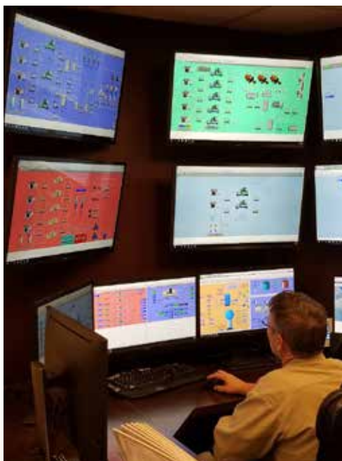
Plant Operator Dennis Pennings monitoring status of all utility plants from inside the newly remodeled control room at Central Plant.
