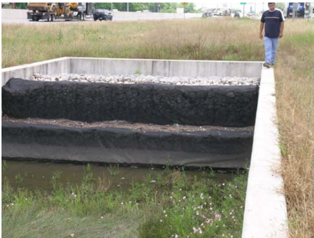
TX DOT highway runoff collection/filtration compartments.
