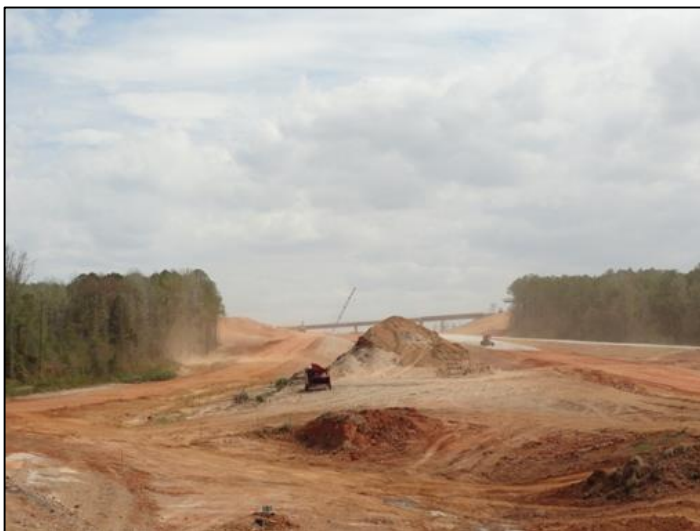
Figure 5 Construction of Toll Loop 49 Segment 5 at Paluxy Drive (TylerTexasOnline Staff photo) (September 2011)
