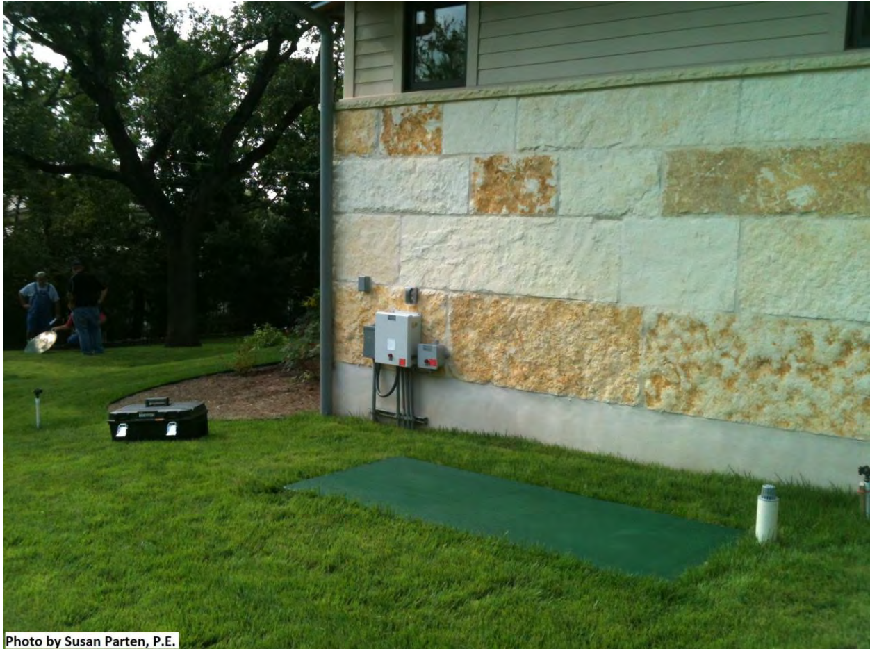
Photo 1: Recirculating media filter unit (closed).
