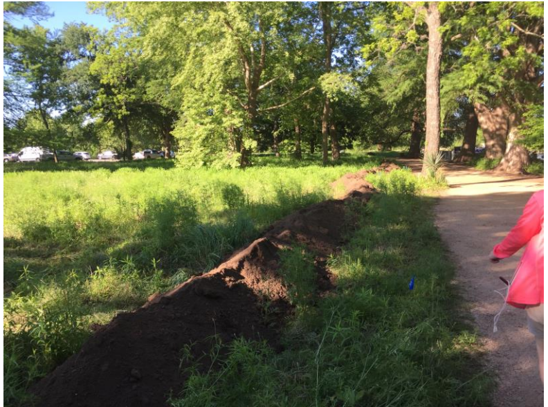
Figure F: Laying out berm soil height adjacent to riparian planting site
