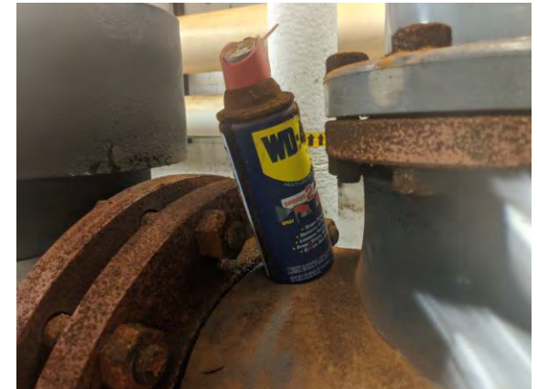
View of general corrosion
