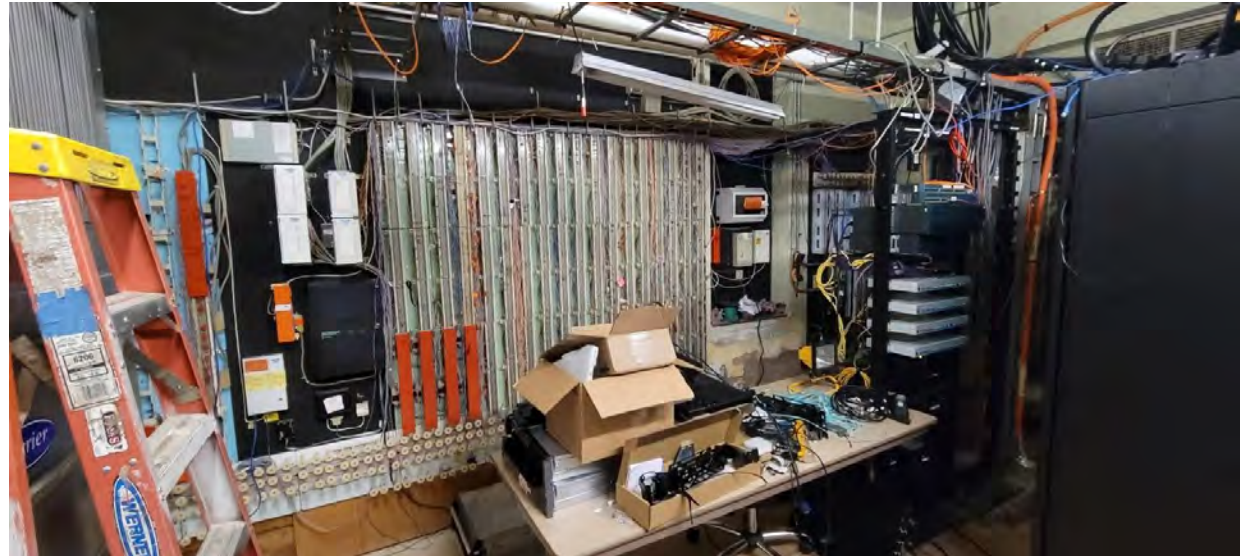
Main server room
