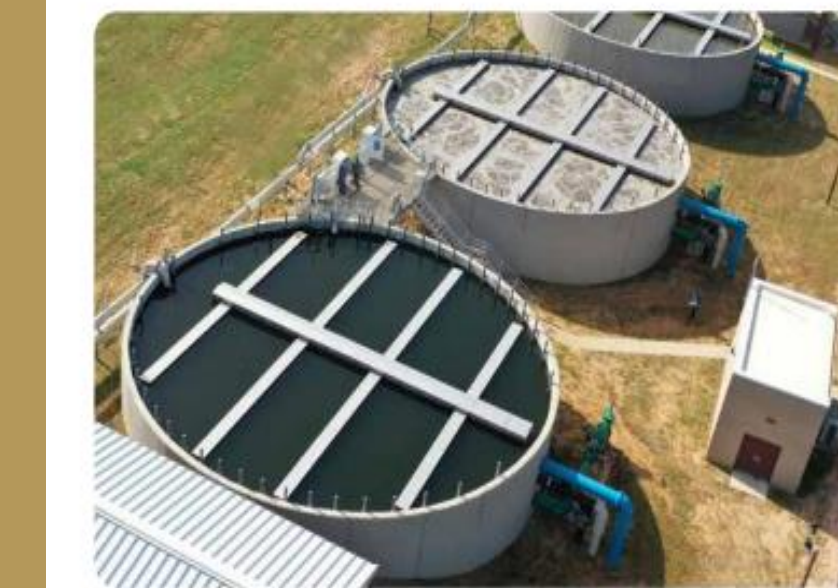
Three AquaNereda ® reactors show compact design, typically 50% of a conventional plant.
