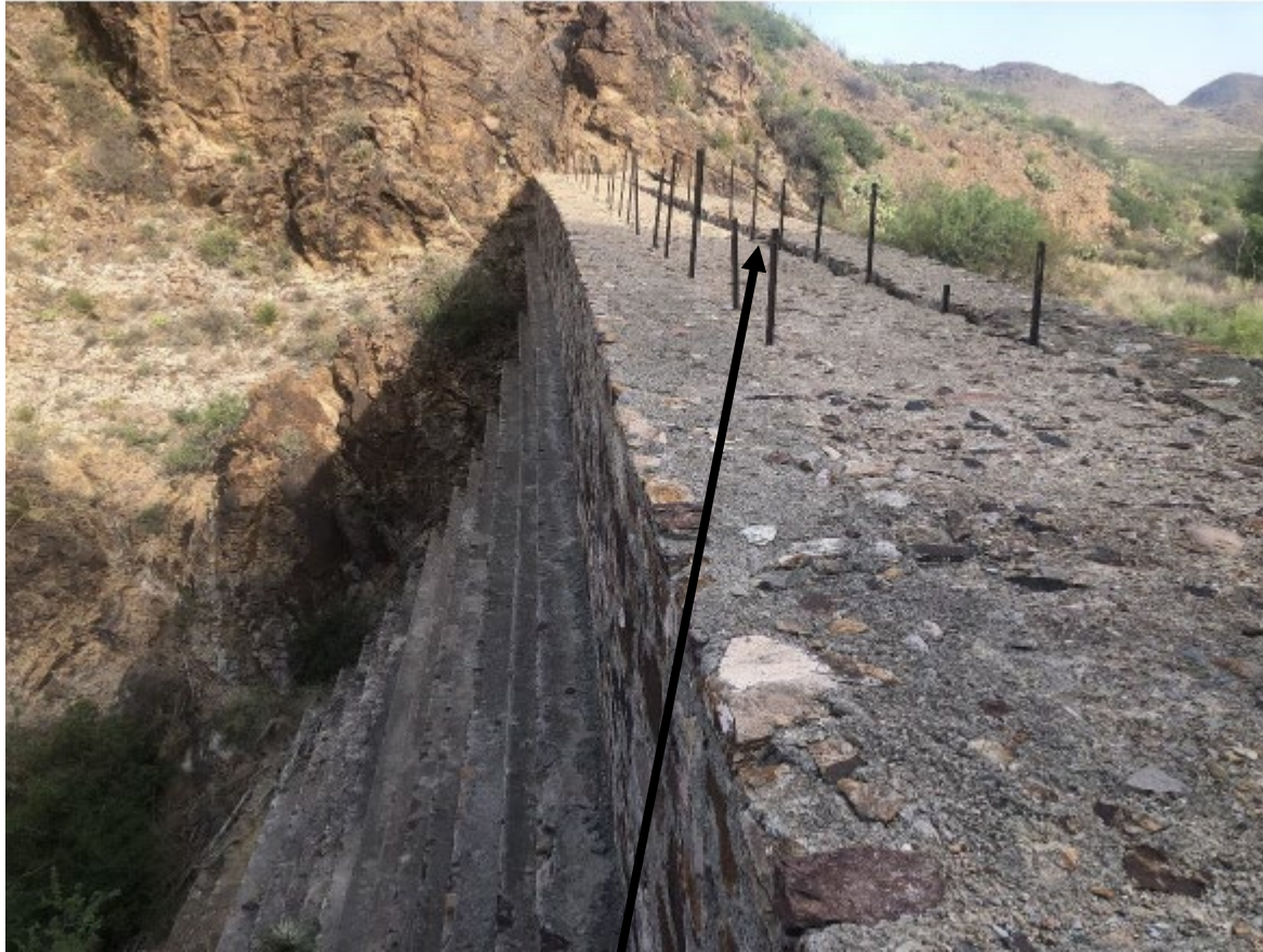
Cracks at top of Dam noted on TCEQ's 2016 Dam Safety Inspection Report
