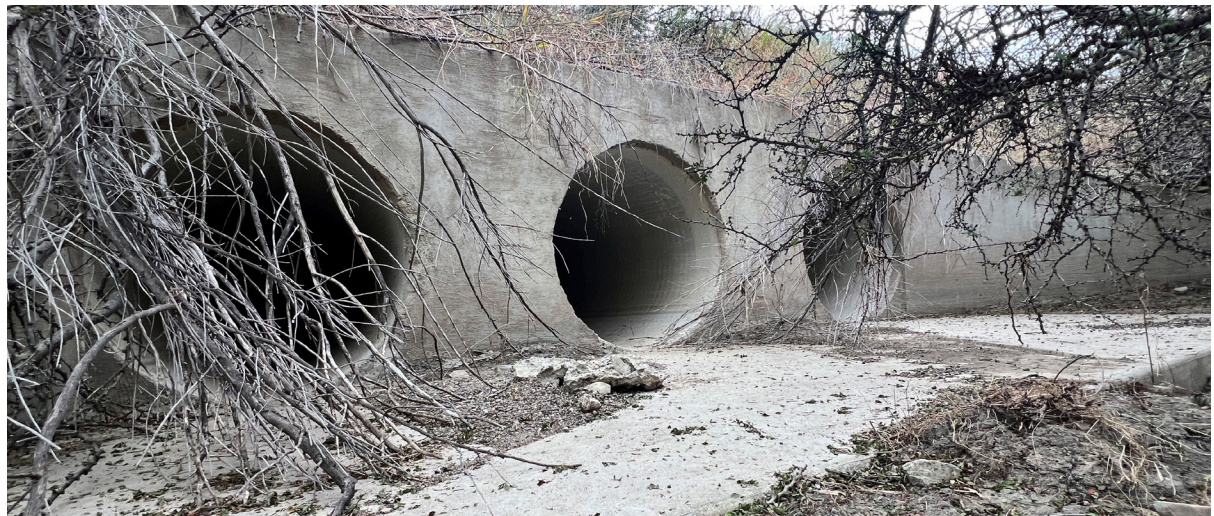
Outfall Pipes Draining Adjacent Detention Basin into SRSU Property
